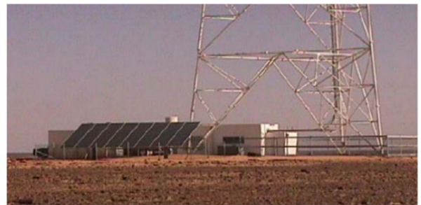
Fig. 6. PV panels installed to supply telecommunication towers [7].
